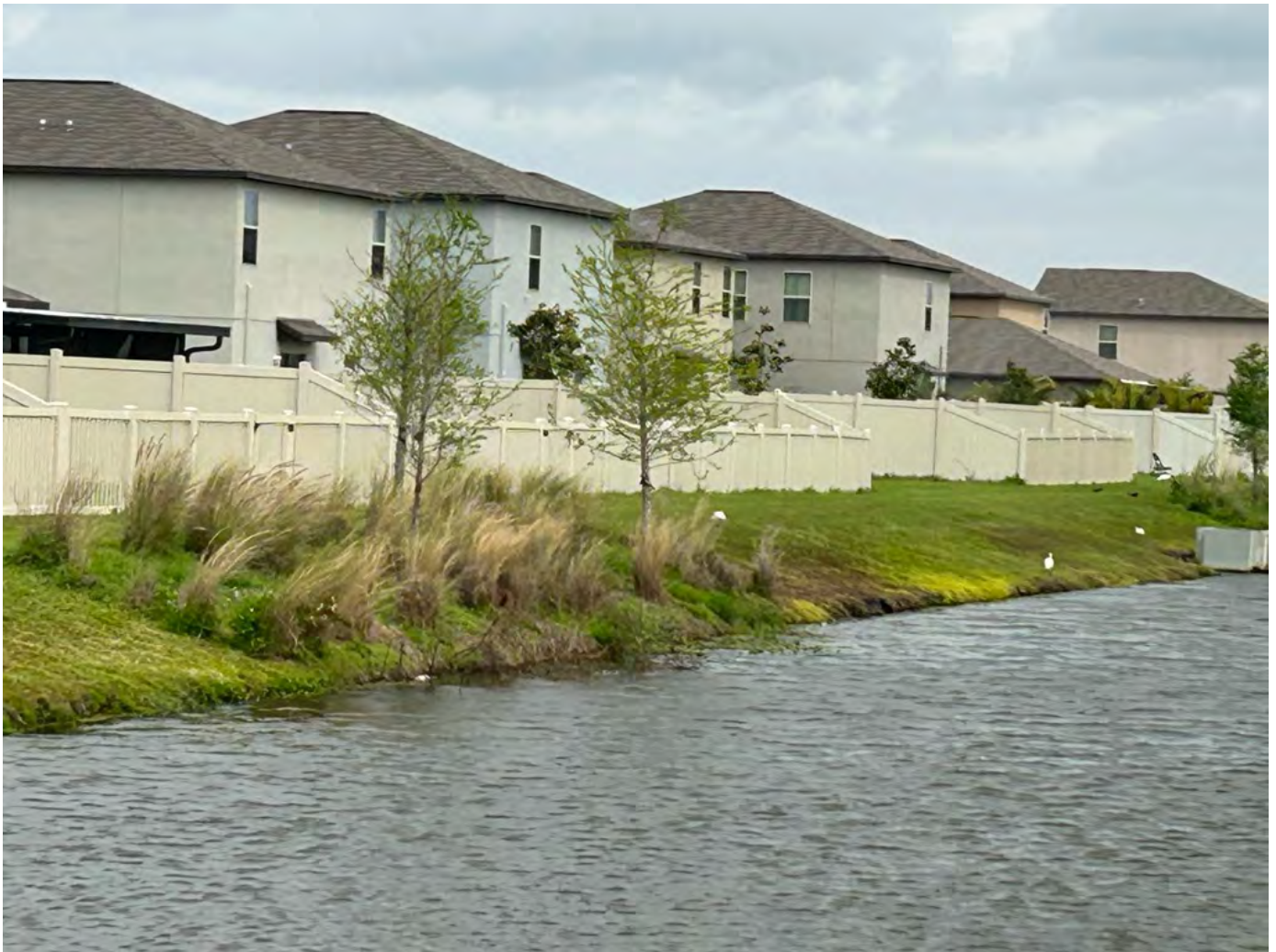
Pond Bank - Area Mowed And Line Trimmed. Grass Bed Is Growing Quickly
